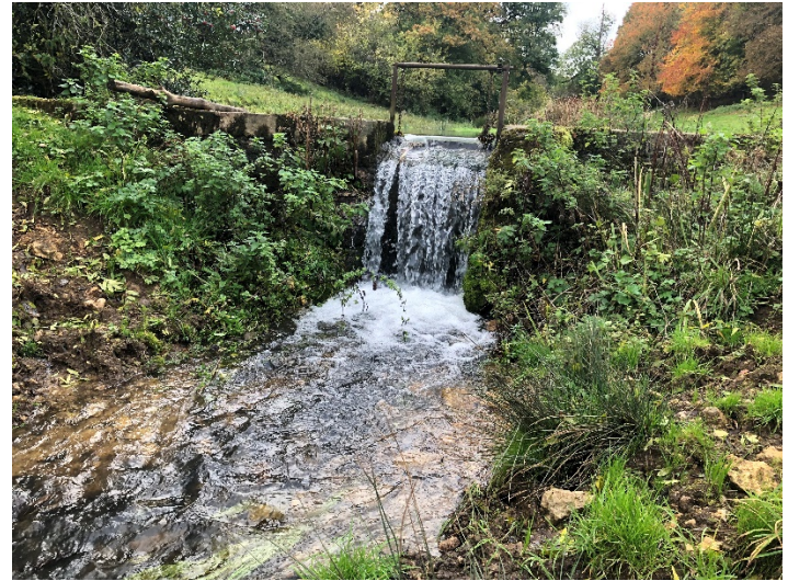
Site 5 – Man made concrete and metal barrier made impassable to migratory fish; except eel
